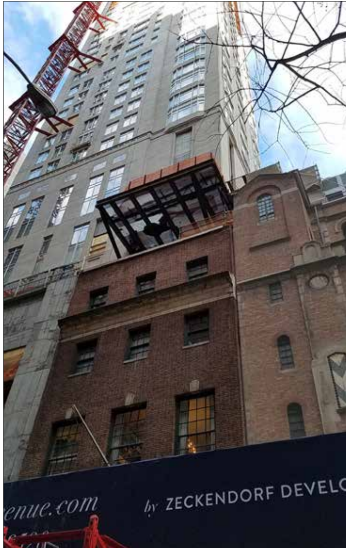
The Grolier Club (the darker brown building with three windows per floor) is now wrapped by a new building (still under construction) to which it sold its air rights for what was reported to be about $7 million.
